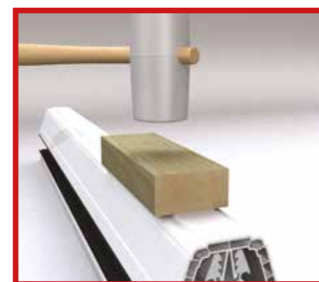
Knock the glazing bar top cappings on with a Deadblow hammer. Greater care is needed in cold weather. Keep all trims wrapped until they are needed. Once again each capping is numbered according to its position in the roof.
