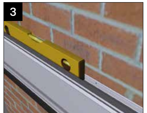
Lift the box gutter back into position, check levels, and then mark the wall (through the pre-drilled holes) ready to drill the host wall and grind out for the flashing.
