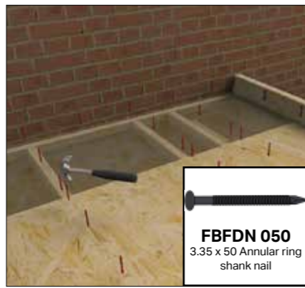
Use the nails provided to secure the board down into the firings at 300mm centres.
