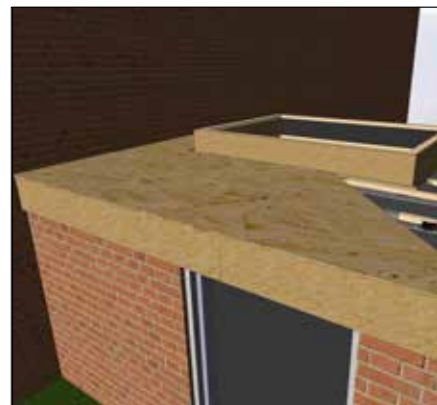
Continue around, gluing and placing until a full section is complete. Note: Boards are oversized at drip edge to be cut back to suit rip detail being fitted.
