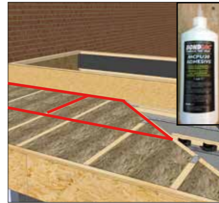
Select the adjoining OSB as per the location plan, glue the joint and position together.
